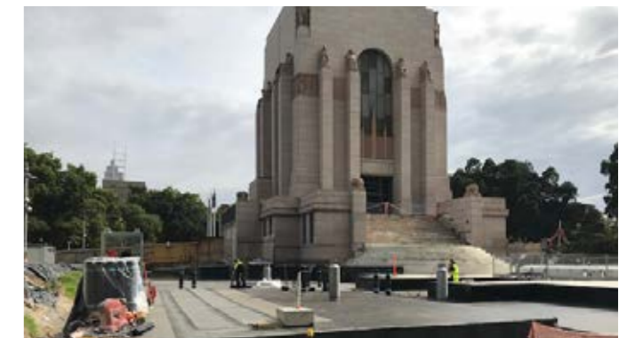
Over 12,000m 2 of TREMproof Torch was used on the water fountains and walkways
