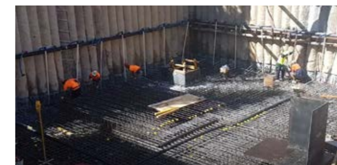
The site was 50 metres from Manly Beach and 4 metres below sea level
